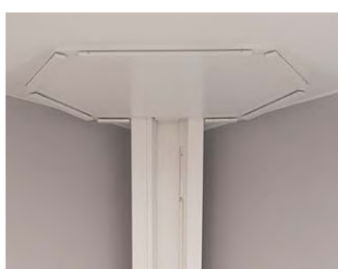
Fire seals for both levels
